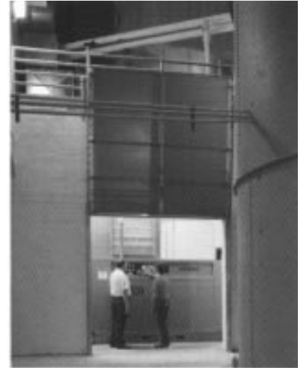
Dave Stewart, Plant Engineer, and Joe LaRocca, Maintenance Electrician, check the Sullair Series 25, 24KT model rotary screw compressor at Ace Hardware Corporation's Paint Division facility in Matteson, IL.
