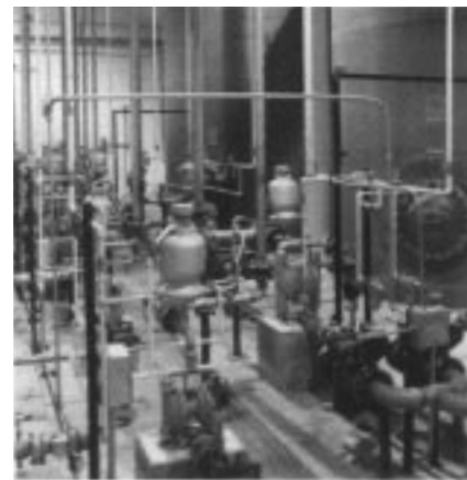
Air diaphragm pumps are used to transport raw materials from storage tanks to mixing tanks, and to convey the blended paint products to the packaging area.
