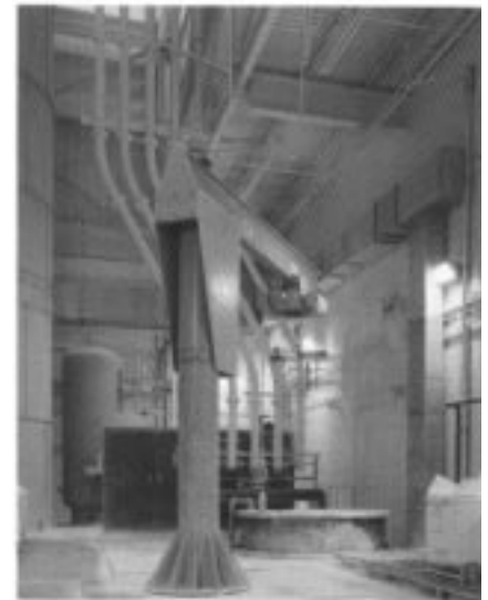
The pigment storage area, showing part of the dense phase pneumatic conveying system for dry powders.
