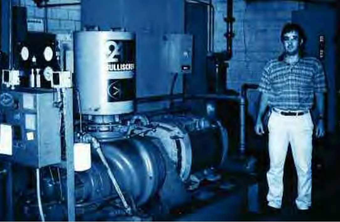
Maintenance and Facilities Engineer Alberto Koett checks a Sullair 24KT™ compressor that has been delivering oil-free air at Caribe GE for more than 25 years.
