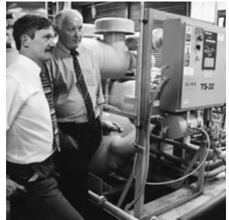
Michael Boland, Plant Maintenance Engineer, and Stan Waldron, QA and Technical Services Manager, with the Sullair tandem compressor that helps save energy at Bourns Electronics.
